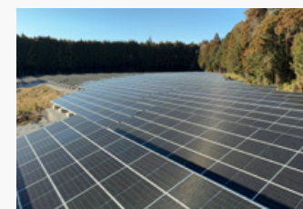
Solar Power Generation System at PDRadiopharma's Chiba Plant
